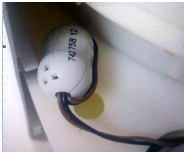
Picture #7 Ferrite installed on the power cable
